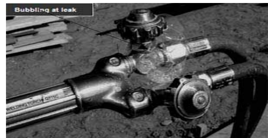
Figure 2. Bubbling at leak
